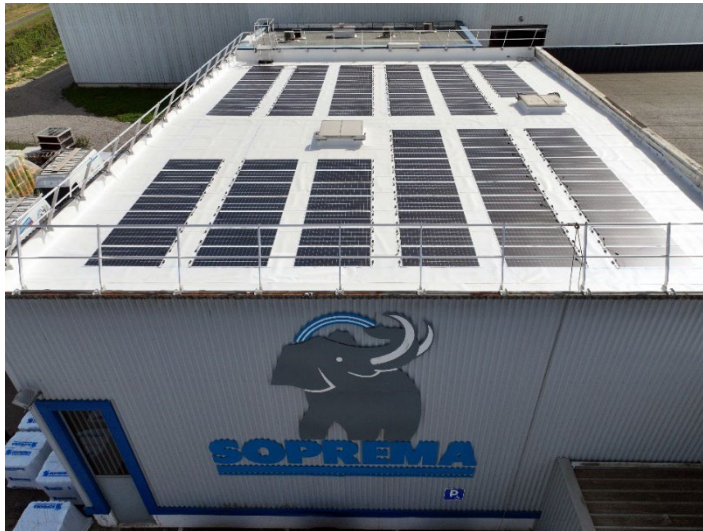
Figure 2. First demonstrator of 22kWc in a Soprema building with STYKON® panels.
